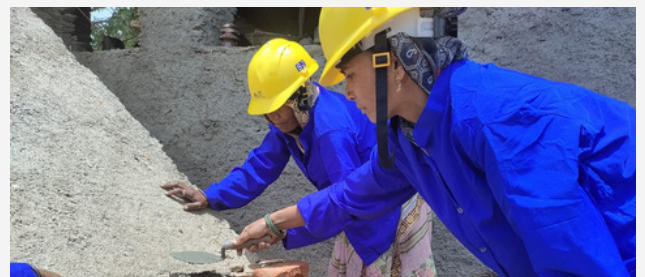
Woman is promoted to Mason from Helper on the construction site after our intervention
